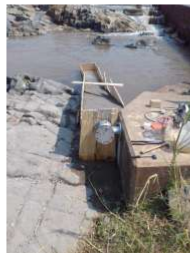
Figure 15: New conduit pipe for the water quality probe, secured to the rock bed using metal rods and concrete
